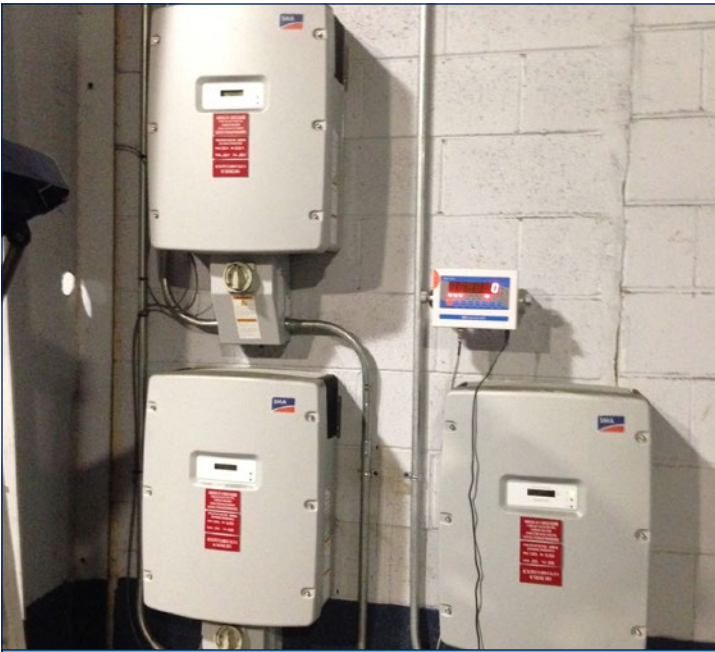
Figure 5: Inverters and a monitor allow power production to be monitored onsite as well as instantaneously online.
