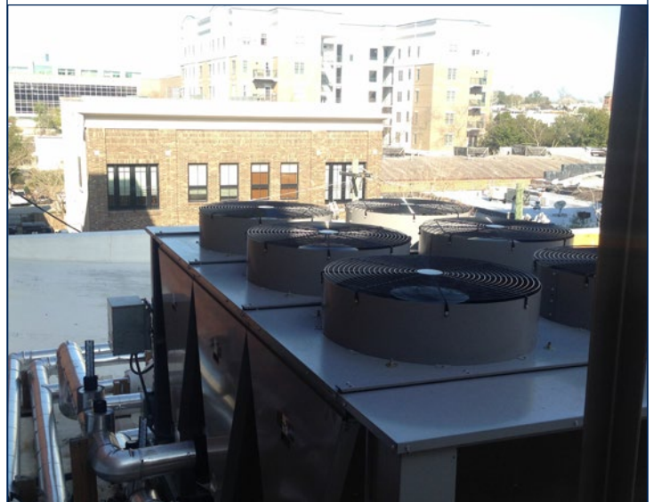
Figure 3: The building's chiller was replaced in 2013.
