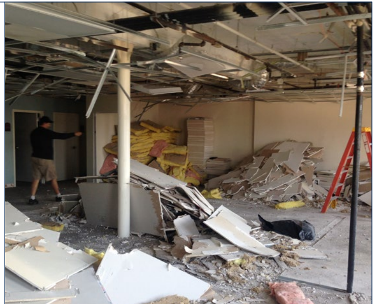
Figure 4: An office suite on the building’s fourth floor will be built out to include energy-efficient lighting and other features.
