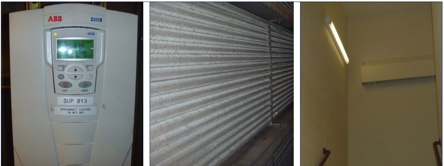
Figure 3: Key components of Biological Sciences' retrocommissioning plan: an installed VFD (left), hot water coils (middle), and a dimmable LED in a stairwell (right).
