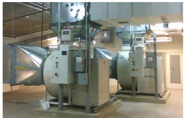
Commercial HVAC systems are fine-tuned during retro-commissioning and assessed for energy improvement opportunities during an audit.
